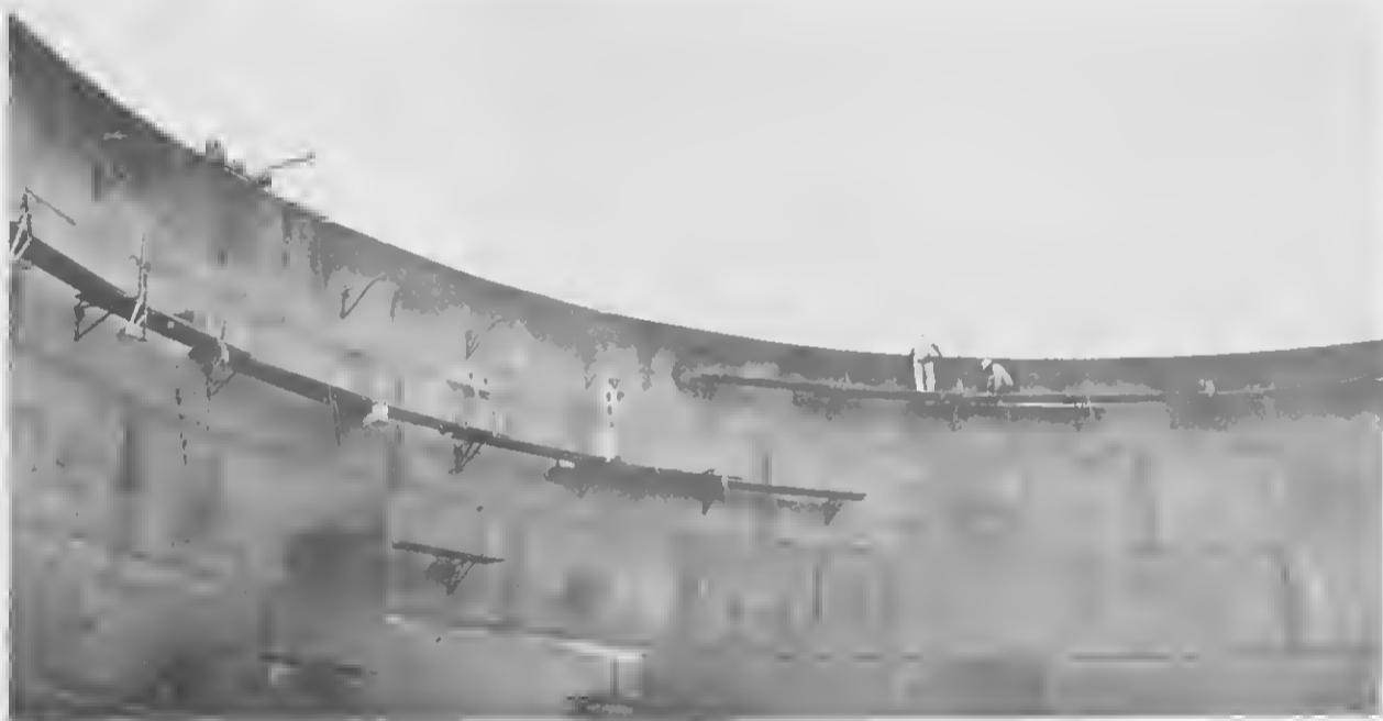
WORKMEN SEEM dwarfed by the tremendous circular sweep of the tank's inner wall. The plates that make up the sides have smaller thicknesses as they approach the top.
